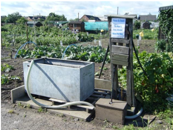
The new installation in front of the historic pump
